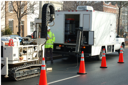
On a jobsite with the Columbia Technologies 6620DT and MIP support vehicle equipped with mobile laboratory equipment.
